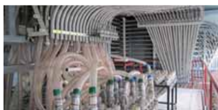
Raw material transfer lines
